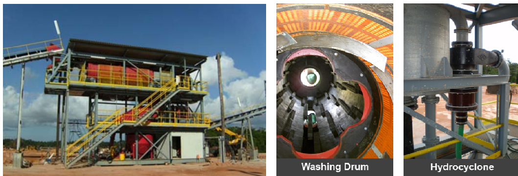
Figure 1. Flow-sheet and pictures of Bauxite processing plant for the removal of reactive silica, planned and delivered from AKW A+V.
